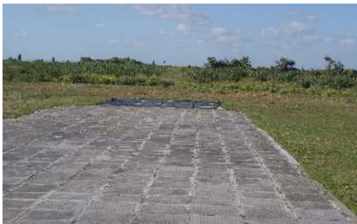
Concrete slab runway may look rough, but is adequate for club's activities.
